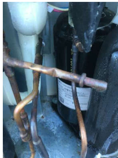
Auxiliary pipe LP & HP
